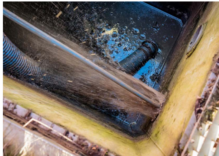
Fig. 13: Sediment being pushed out of the channel into the well
